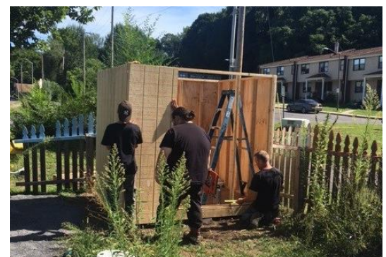
Ulster Youth Build created a tool shed at Rondout Garden, coordinated by a H&W project manager
