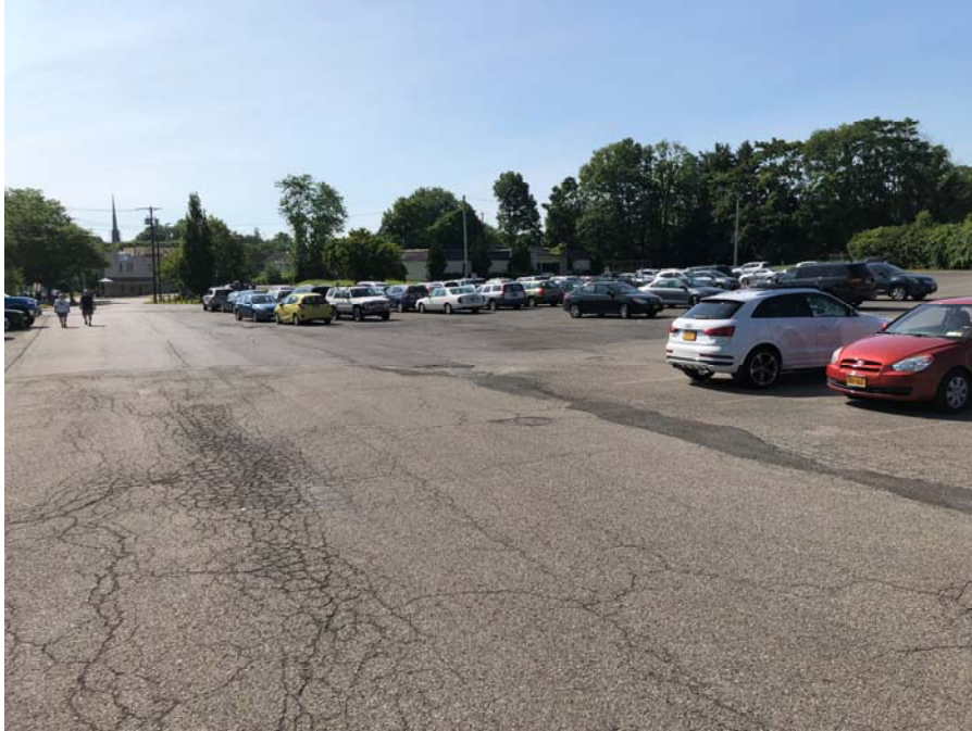
Overall picture of parking lot showing cracking and patches
