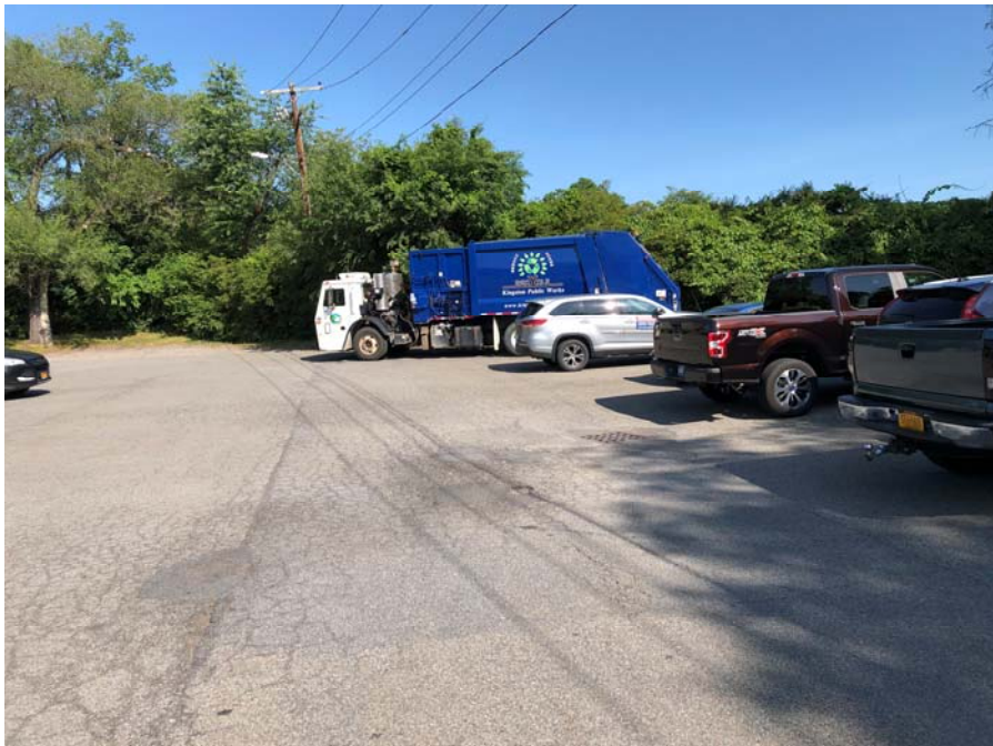
Picture of asphalt at drive isle showing cracking
