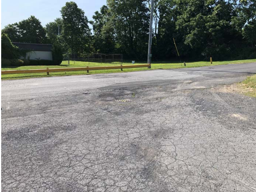
Picture looking at Severyn Street showing pavement cracking
