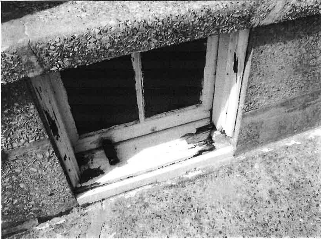
Evidence of rot at wood window frames.
