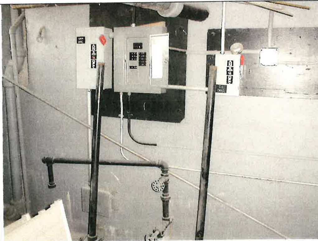
Existing electrical service – 100 amp panel and disconnect switch.
