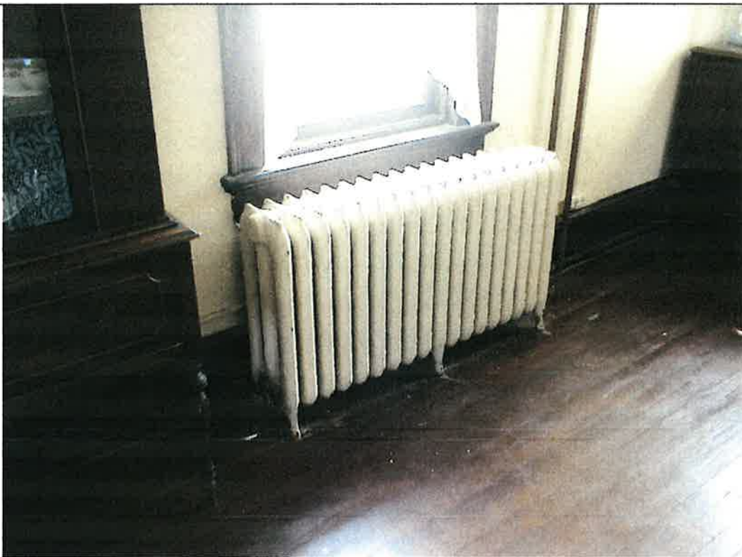
Existing Heating System – Boiler, Oil Storage Tank (top) and typical radiator (above).
