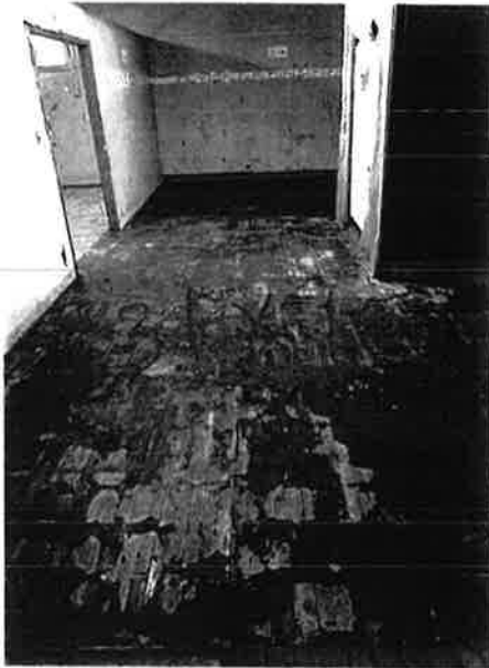
(Left): 31x15 9x9 tile on top of Non-ACM Tar-paper Mastic
